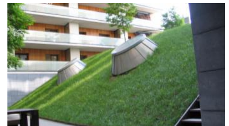
The pitched roof shortly after installation of the turf. Skylights allow for natural daylight inside the building.
